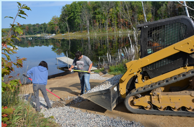
Filling in the sides with riprap rock to help drain water and prevent erosion
